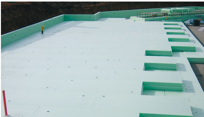
Fig. 39: The second insulating layer, likewise of Styrodur boards with shiplap edges, is laid with the joints offset to the first layer of boards and also in a loose bond.
