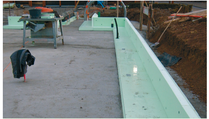
Fig. 34: The arrangement and installation of linear edge elements is performed on the flat base according to the respective building installation plan.
