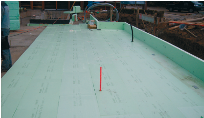
Fig. 38: The Styrodur boards with shiplap edges are laid in a loose bond in the first insulating layer. The point at which the installation begins and the laying direction is planned for the individual building and crafted to the assembly plans.
