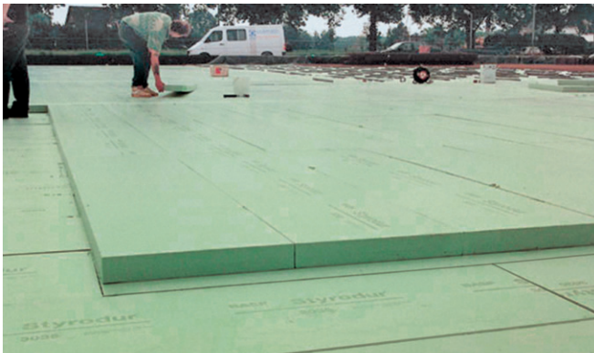
Fig. 8: Multi-layer installation of Styrodur boards under a floor slab according to DIBt approval Z-23.34-1325.
