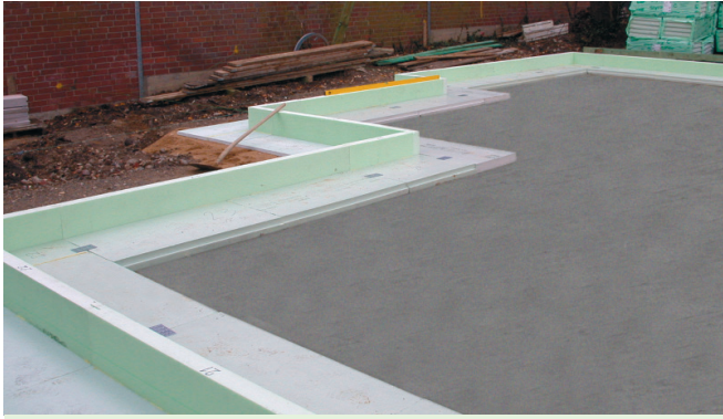
Fig. 37: Frost protection in accordance with EN ISO 13793 is necessary to avoid an expensive foundation extending down to the frost depth. It is added to the edge element in the factory and deployed as part of the horizontal ground insulation.
