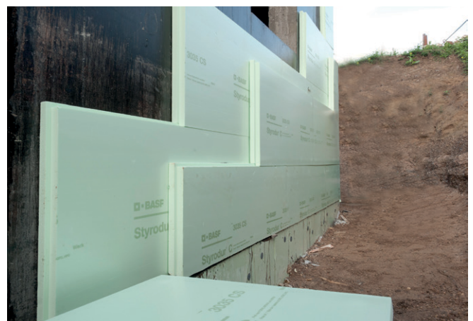
Fig. 3: Securing a two-layer perimeter insulation of Styrodur boards until the backfilling of the excavation pit.
