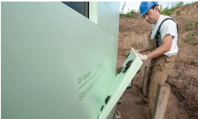
Fig. 5: Point bonding the second layer of Styrodur boards with shi lap and offset joints.
