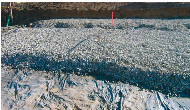
Fig. 33: A gravel bed as a blinding layer and levelling plane makes for a flat base. This base course is prepared and compacted in line with the requirements of the building ground and the instructions of the structural engineer.
