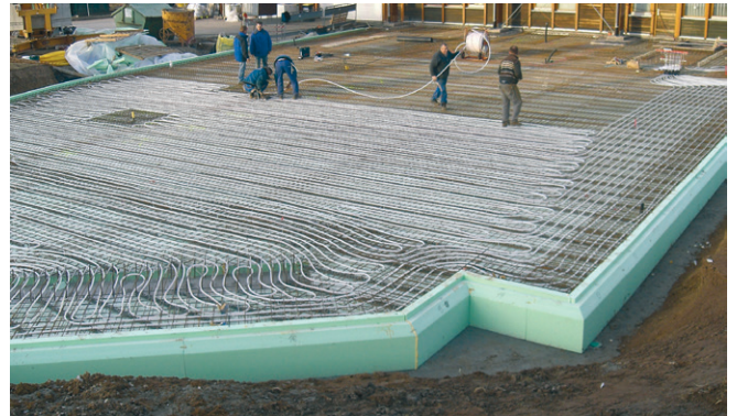
Fig. 41: The thermally active floor slab serves as a large-scale heat accumulator and yields energy savings of up to 30 %. The reduction of the floor structure provides additional room height.
